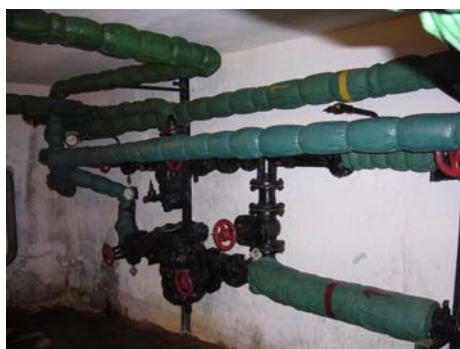
Existing heating point connection
