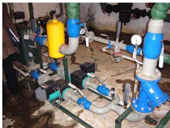
Example of new substation connection with heat exchanger
