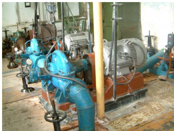
Water distribution pumps
